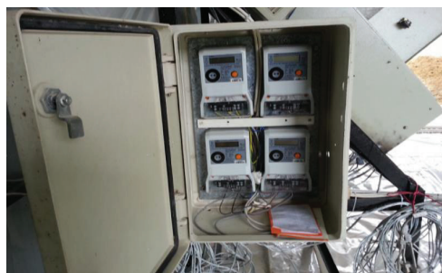
Figure 10. Electric meter counter to determine energy consumption by aeration fans
