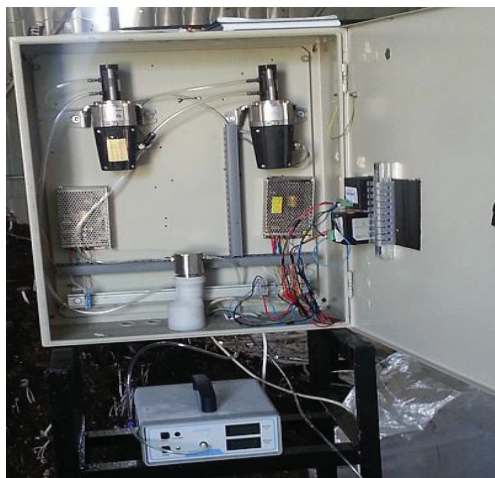
Figure 8. Gas measuring unit
