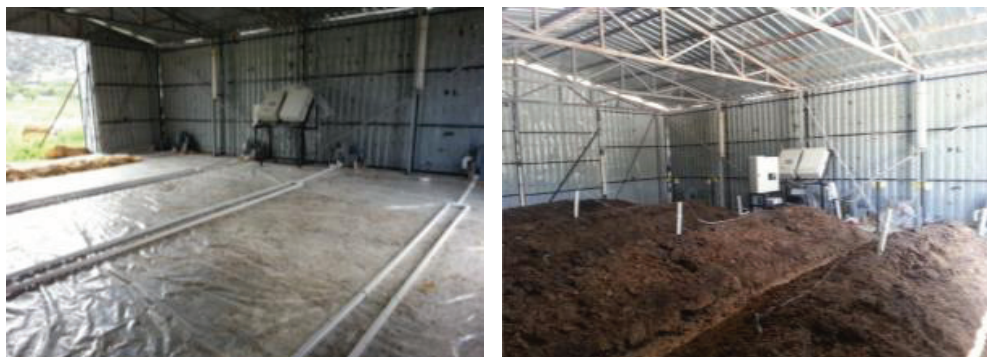
Figure 1. The pilot scale aerated static pile composting systems
